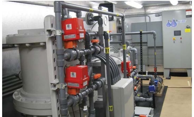
One of two 90 gpm FilterSure filtration units. Electrical control panel is shown in the background.
